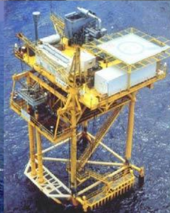
Wellhead platform (B, D, WSD)
